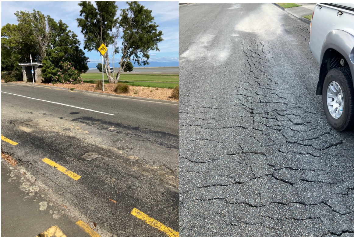
Figure 8-19-2: Pavement failures on bus routes
