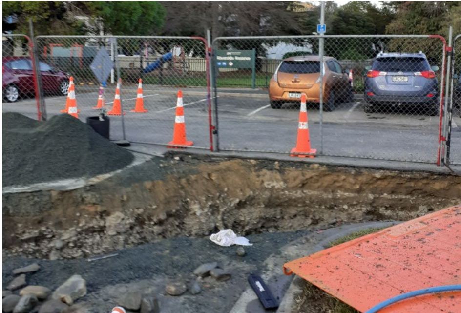
Figure 8-3-2: Clay pavement layer below the seal layer is revealed in a utilities trench (Riverside Drive)
