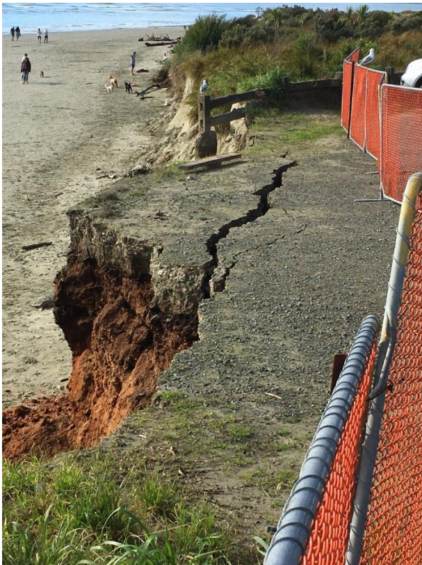
Figure 42: Erosion at Tāhunanui Back Beach, May 2023
