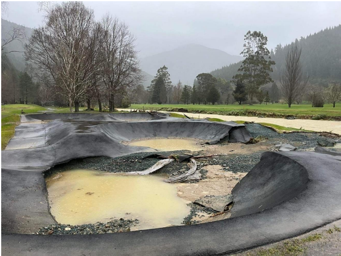
Figure 37: Maitai Pump Track immediately following August 2022 weather event
